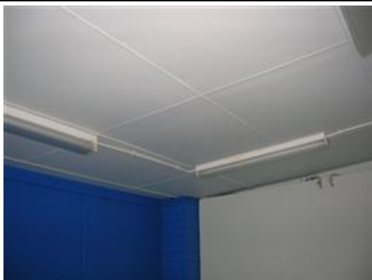
Photo No: Photo-12 Feature: Ceiling Material: Flat cement sheet Location: Western Beach Road; Building: RX; LEVEL 1; Room: RX.02 Sample Reference: 69311-13 Item Status: Positive
