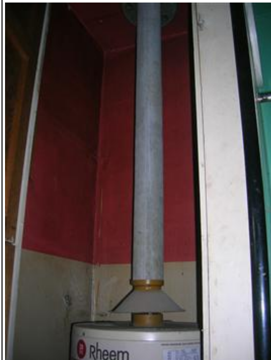
Photo No: Photo-04 Feature: Hot water service Material: Moulded fibro cement flue Location: Western Beach Road; Building: 92-94; WESTERN BEACH RD - LEVEL 2; Room: BR.19 Sample Reference: 69311-9 Item Status: Positive
