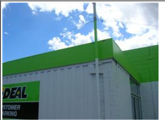
Photo No: Photo -15 Feature: Fascia Material: Flat cement sheet Location: Western Beach Road; Building: RX; Level: External; Room: External Sample Reference: 69311-15 Item Status: Positive
