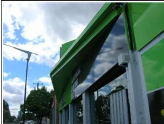
Photo No: Photo-16 Feature: Porch Ceiling Material: Flat cement sheet Location: Western Beach Road; Building: RX; Level: External; Room: External Sample Reference: Similar To 69311-15 Item Status: Assumed Positive
