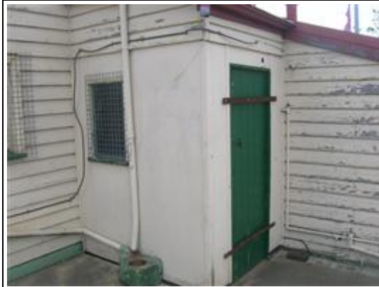
Photo No: Photo-07 Feature: Wall Material: Flat cement sheet Location: Western Beach Road; Building: 92-94; Level: External; Room: External Sample Reference: 69311-12 Item Status: Positive
