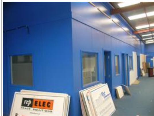
Photo No: Photo-13 Feature: Wall Material: Flat cement sheet Location: Western Beach Road; Building: RX; LEVEL 1; Room: RX.01 Sample Reference: 69311-14 Item Status: Positive
