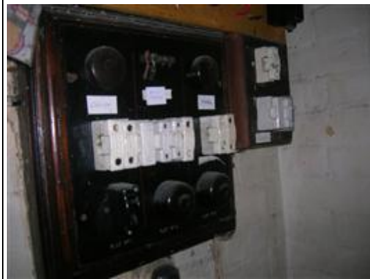
Photo No: Photo-11 Feature: Switchboard backing Material: Millboard Location: Western Beach Road; Building: 92-94; WESTERN BEACH ROAD - LEVEL 1; Room: BR.09 Sample Reference: No Sample Taken Item Status: Assumed Positive
