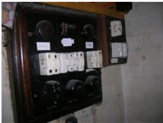
Photo No: Photo-00 Feature: Switchboard backing Material: Compressed cement sheet Location: Western Beach Road; Building: 92-94; WESTERN BEACH ROAD - LEVEL 1; Room: BR.09 Sample Reference: No Sample Taken Item Status: Assumed Positive
