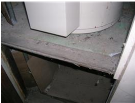
Photo No: Photo-03 Feature: Hot water service Material: Compressed cement sheet Location: Western Beach Road; Building: 92-94; WESTERN BEACH RD - LEVEL 2; Room: BR.19 Sample Reference: 69311-10 Item Status: Positive
